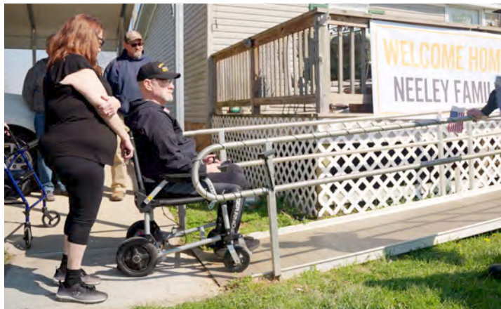
John Neeley can now easily access his home thanks to a ramp and reinforced subflooring which also repaired several holes in the floor.
